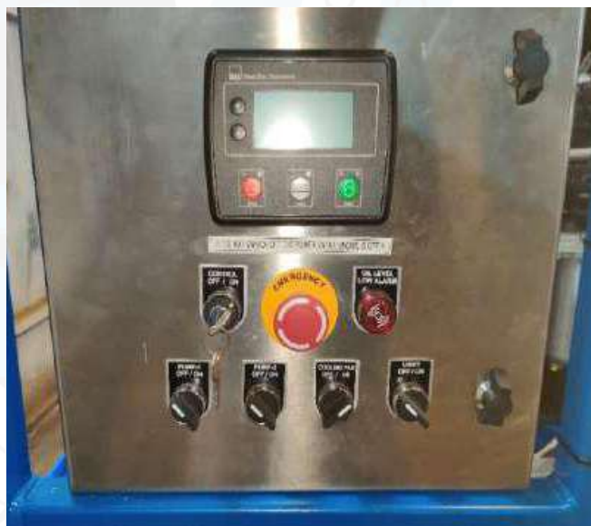
ENGINE CONTROL PANEL
